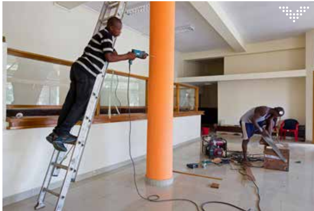
The end of the fitting-out of the new TMB branch in Kananga
